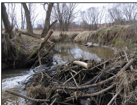
Fot. 12. Zdewastowana tama szósta (fot. P. Brzuski) Photo 12. The sixth dam – after it was vandalised
