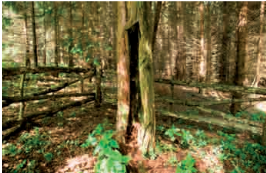
Fot. 3. Zgnilizna brunatna na pniu cisa, drzewo nr 16 (fot. J. Adamczyk) Photo 3. Brown rot on the trunk of yew, tree no. 16
